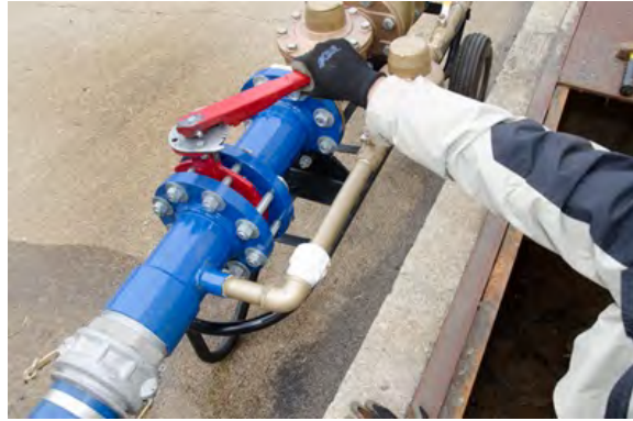
Figure 10 – Back Flushing the Meter
