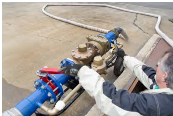
Figure 14 – High Side Valve on Reference Meter
