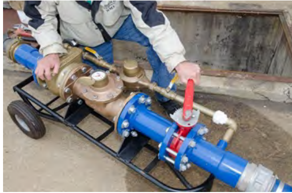
Figure 6 – Purge Air from Test Setup
