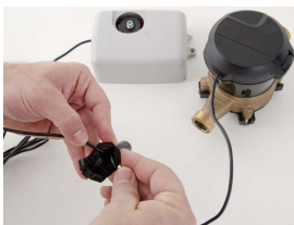
Figure 15: Gray Wires in Slot
