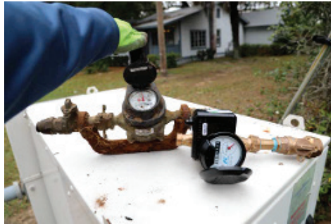
Previous damaged meter next to new Neptune meter
