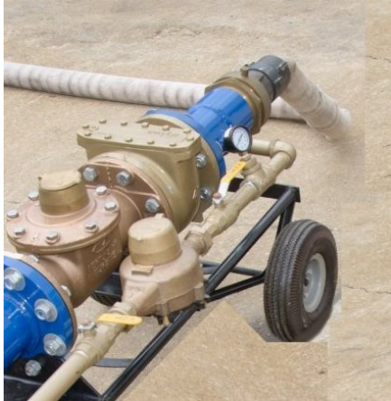
Figure 8 Hose Connection on Reference Meter
