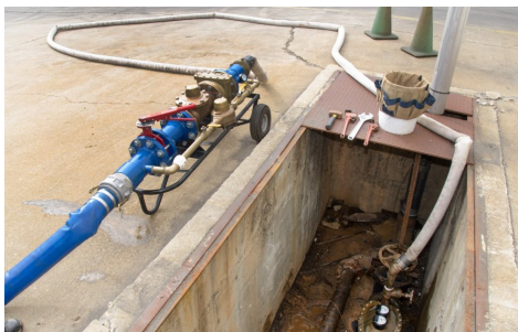
Figure 12 Filling the Test Equipment
