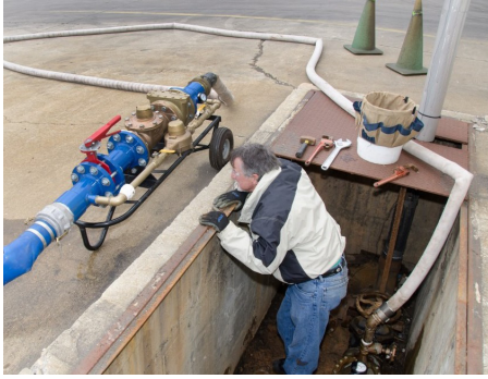
Figure 14 Viewing Inlet Pressure Gauge
