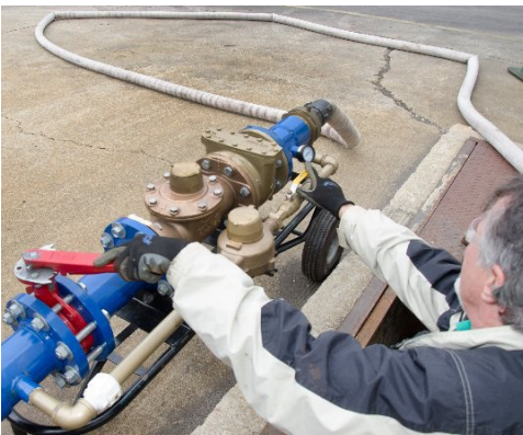
Figure 29 High Side Valve on Reference Meter
